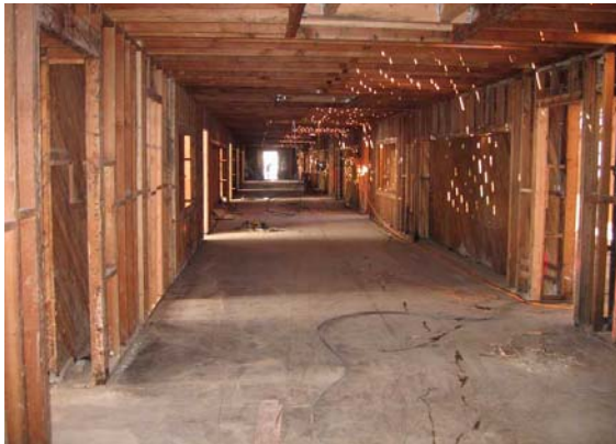
Helix Charter HS – Bldg. 10 Center Hallway
