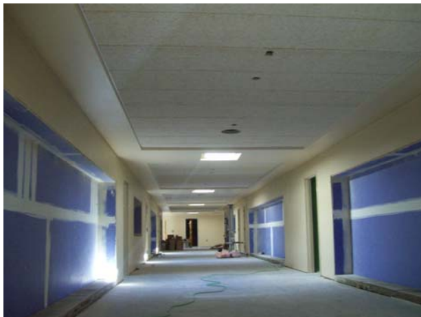
Corridor Lockers & Acoustical Ceiling Tile
