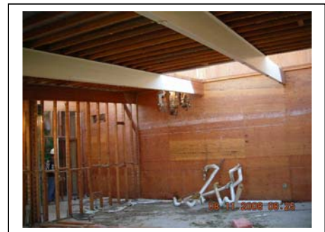
Demo in Building 800
