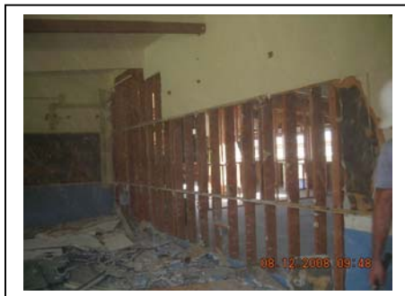
Demo in Building 800
